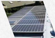
Solar Panel Structure
